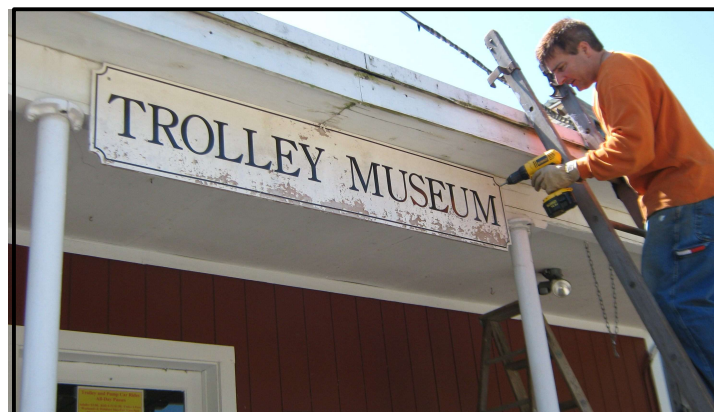
Dave Goff prepares for porch demolition (See Page 5 for what happened next)
