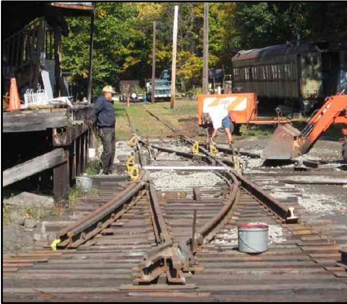
The track department completed the second of the two new turnouts for the carbarn project.
