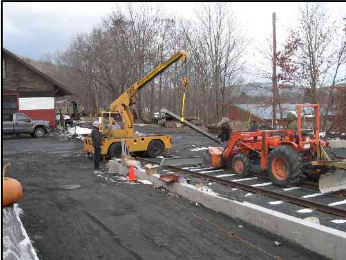
Here we see the first 16-ft cornerpost being hoisted by our own Drott crane.
