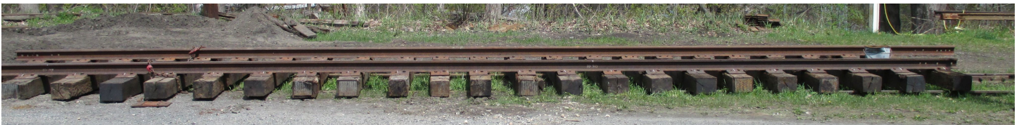
A new panel of track sits temporarily on the House Track. The same panel is shown above on the right, beyond the cones. Soon we will slide it along the House Track rails and into the trench.
