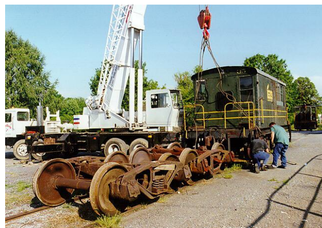
Craning No. 35 from powered trucks to un-powered trucks, so the powered trucks can go to SFTM
