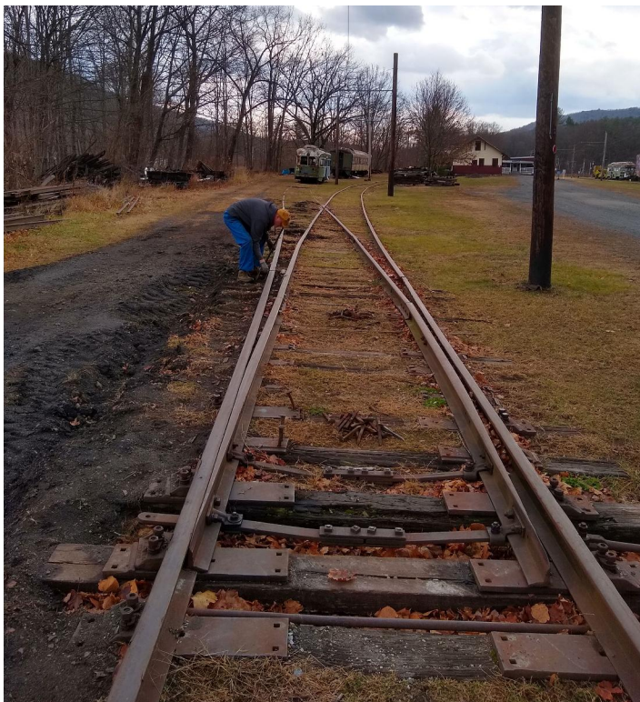
Nash removes bolts in preparation for rail and tie replacement on Turnout 3
