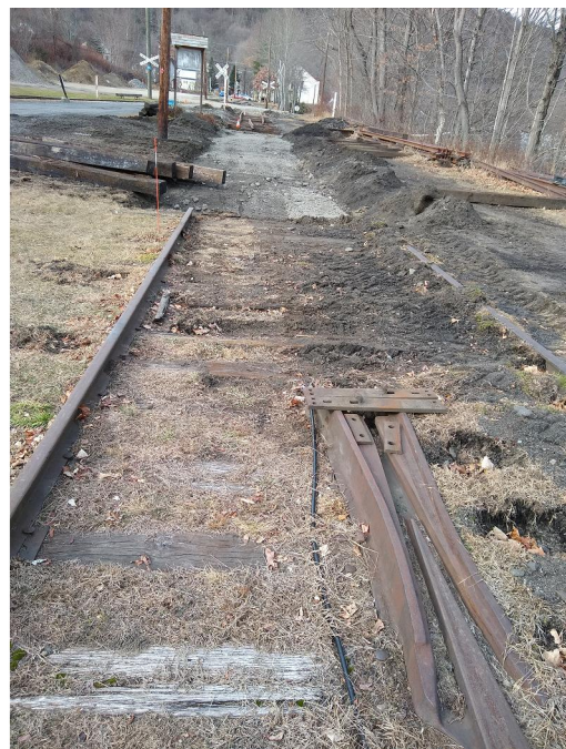
The view looking west from Turnout 3 with ties and rails removed and new sub-ballast in place
