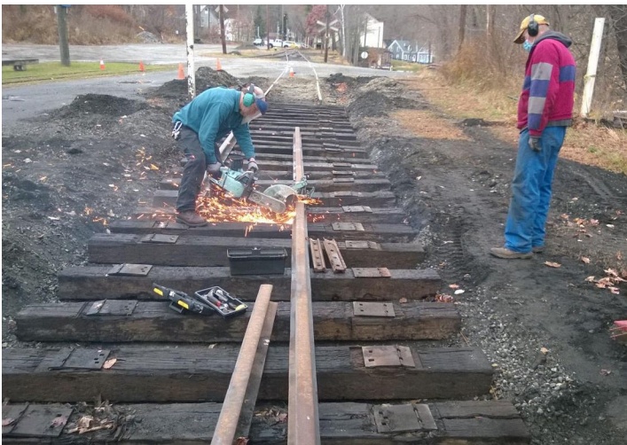
Sam and Nash cut replacement rail to the desired length for the House Track upgrade project
