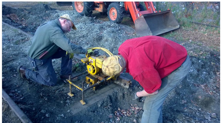
Sam and Nash prepare the rail drill to make bolt holes for the new joints on the House Track. This machine takes longer to set up than it does to drill the hole.
