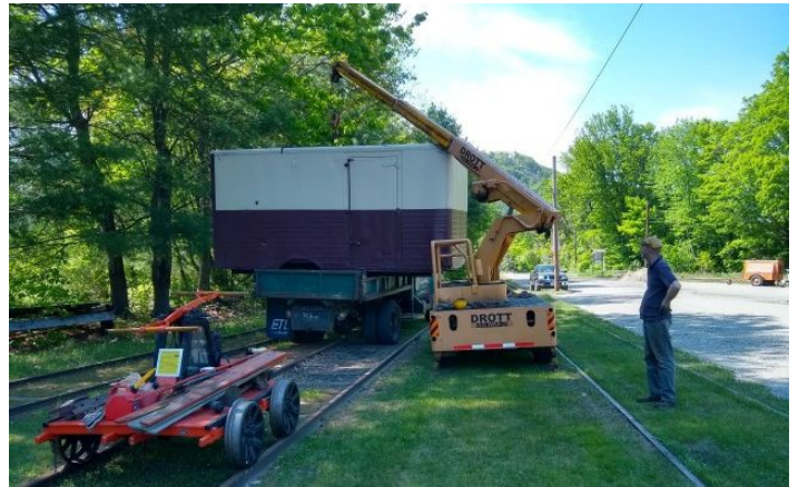
Nash inspects his handi-work after loading the track car shanty onto the boom truck. The shanty has been moved to the east end of the Middle Track.
