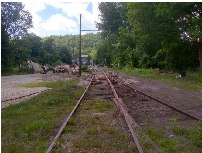
Turnout 3 is ready for House Track traffic. A closure rail for the North Track will be installed later.
