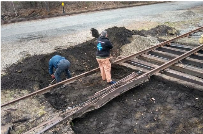
Dave V and Martin prepare the roadbed for new timbers under the frog of Turnout 3.
