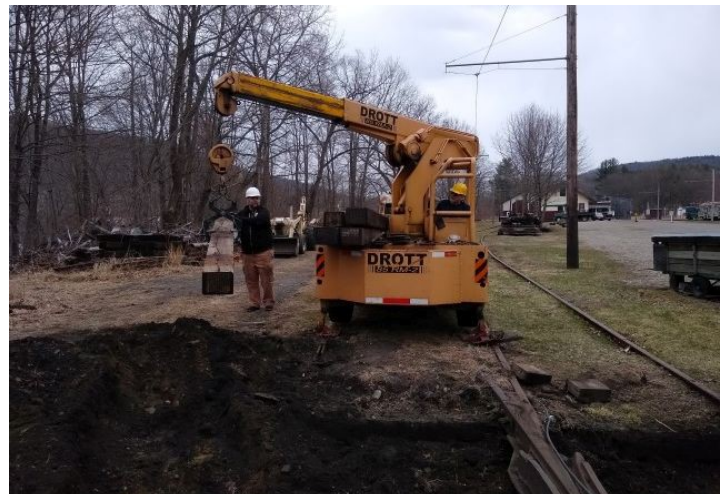
Dave V and Martin use the Drott crane to put a very heavy switch timber in place.
