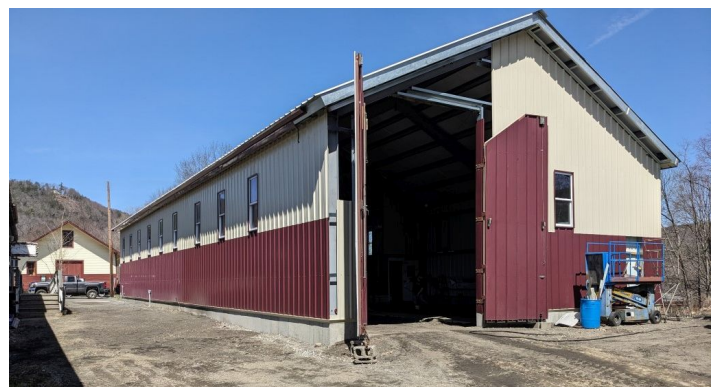
April 2024 - The extended Car Barn is mostly enclosed. The big end doors are hung and operable.
