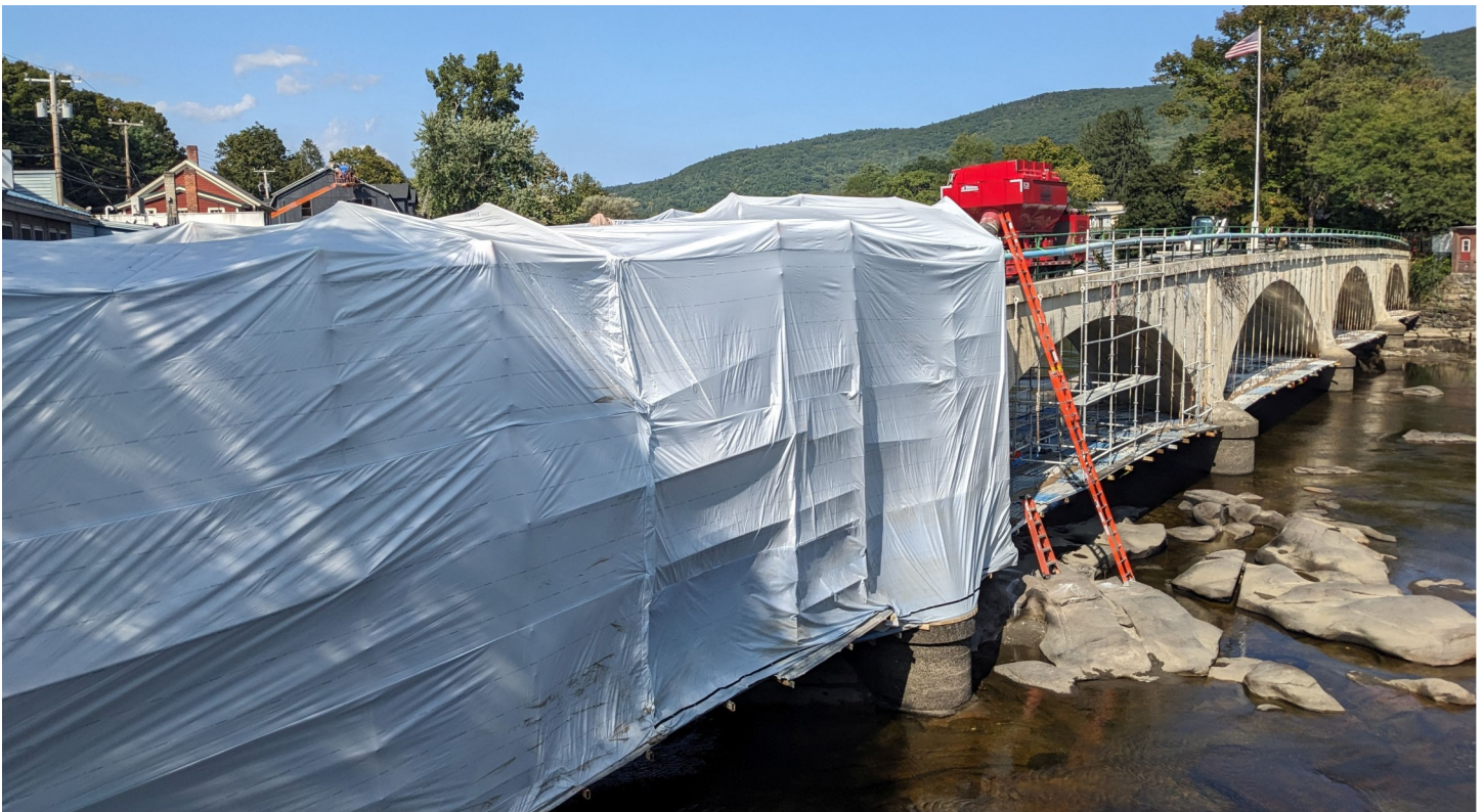
This is how it looks in September 2024. The bridge was started in late July 1908. The first trolley car crossed it in early November 1908. How long will it take to renovate a bridge that was built in less than four months?
