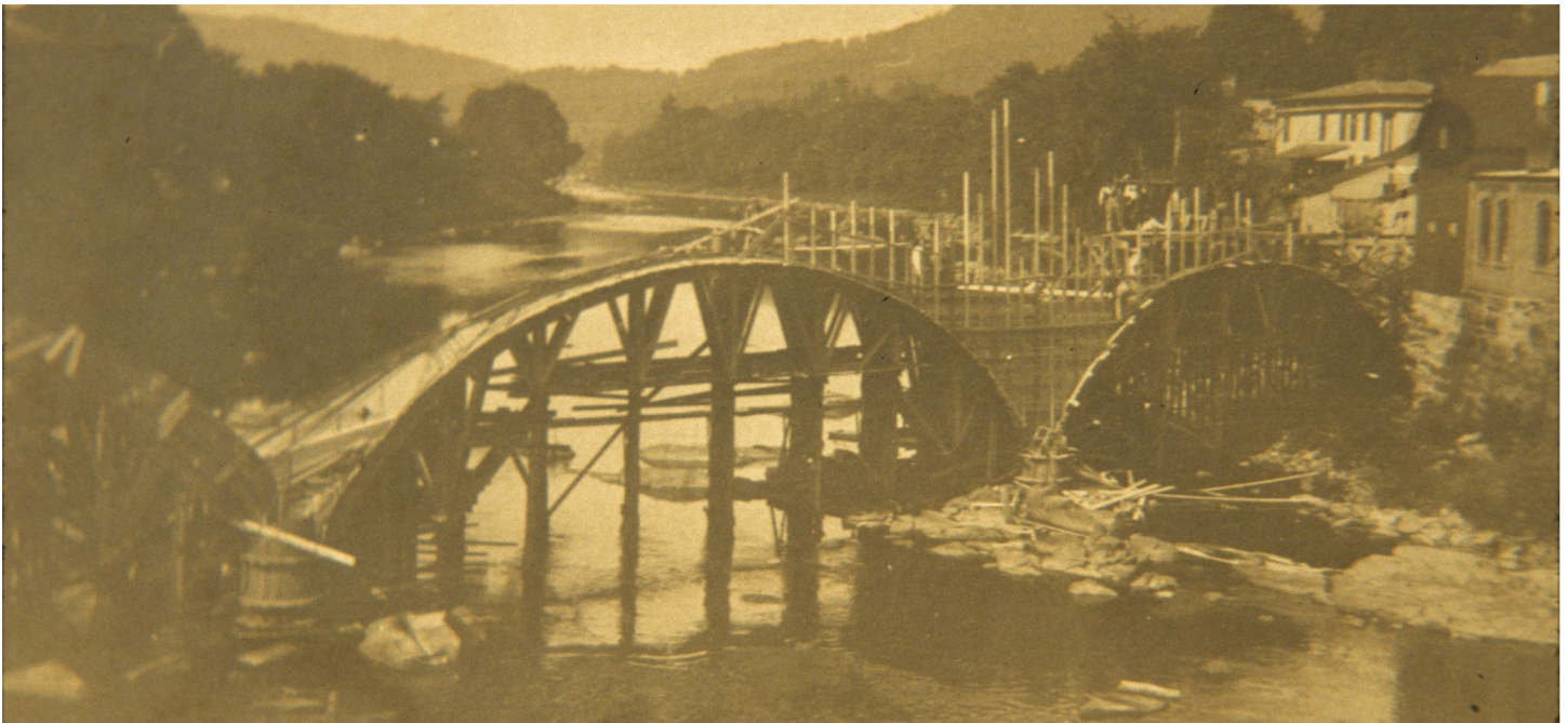
Here is the concrete trolley bridge under construction in September 1908. From Colrain Historical Society.
