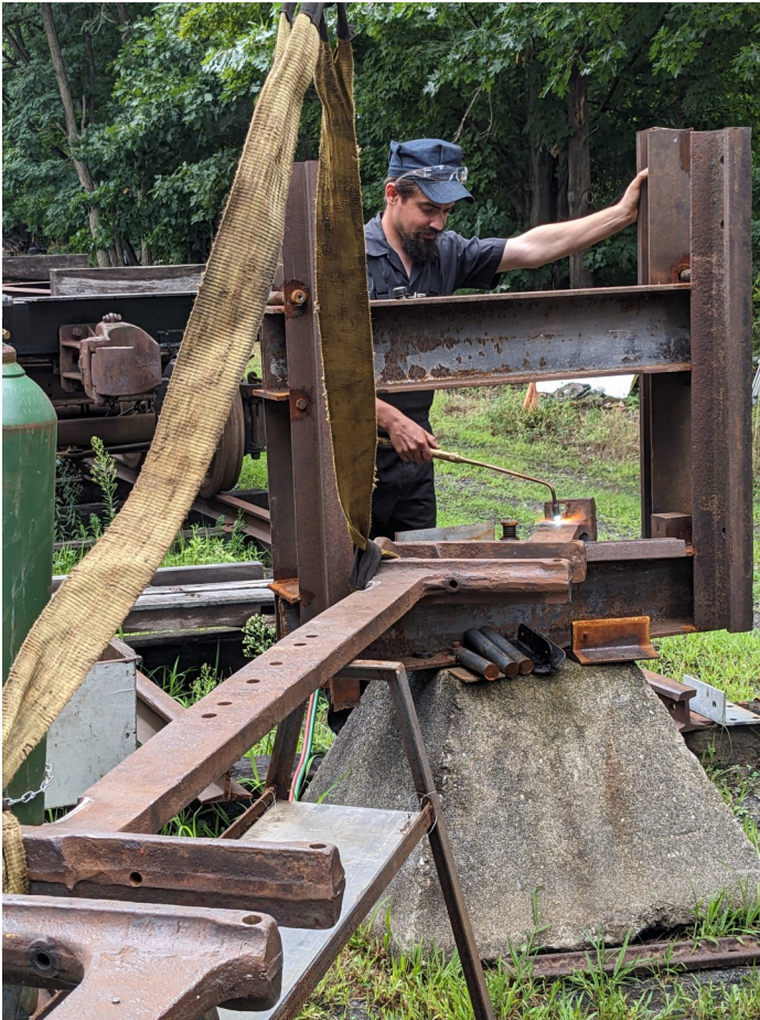
Aug 2024 Josh is heating a bent "Berkshire Hills" truck side-frame in preparation for straightening.
