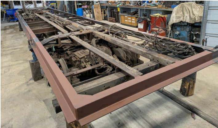
The rotted steel frame members have been replaced and priming and painting have begun.
