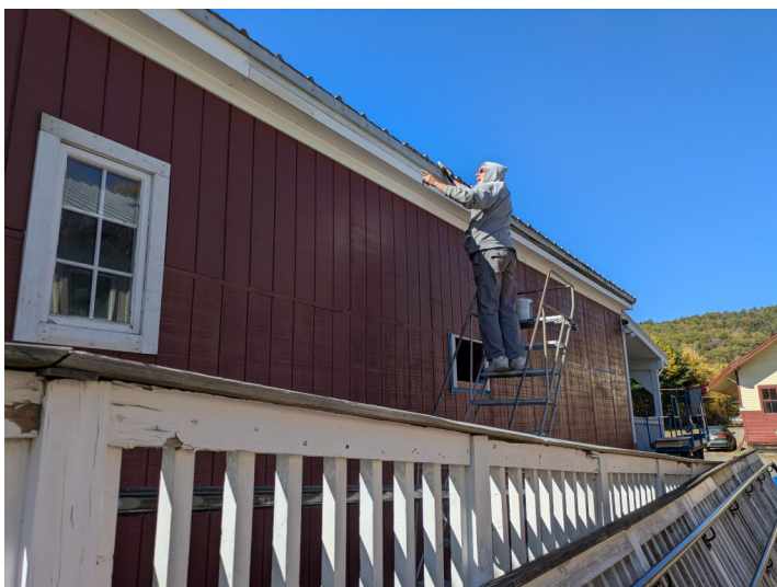
Dick paints the trim on the newly-rebuilt wall. The two old windows were replaced with one insulated window.
