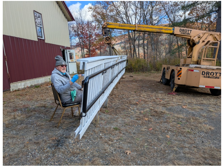
Dick uses the Drott crane to make painting both sides of the ramp railing easier. We had to remove the railing in order to access the wall.
