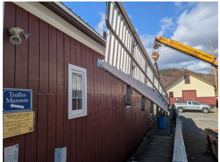
The Drott crane has been very useful. Here it easily replaces the ramp railing after Dick painted it.
